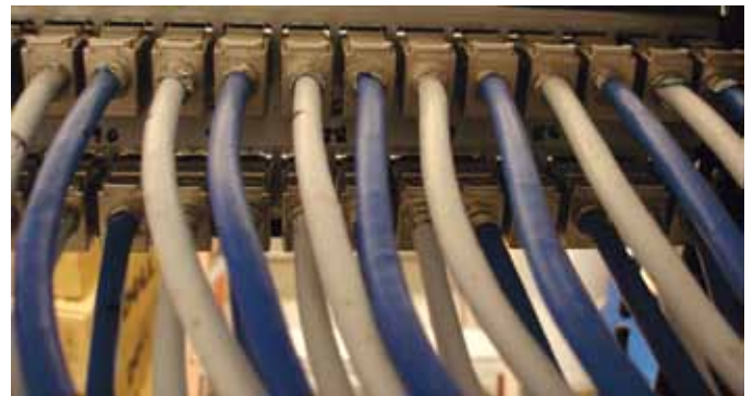
Space savings and improved heat dissipation are two of the benefits Comcast has realized.
